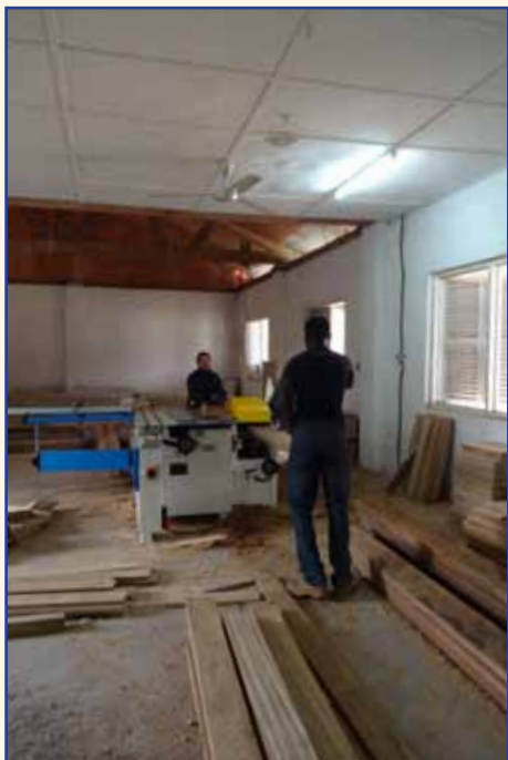
Canon Fragelli cutting the wood that will be used to build the new chapel.
